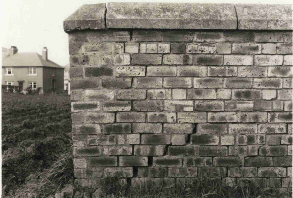
PLATE 4.2. DAMAGE DUE TO COMPRESSION
