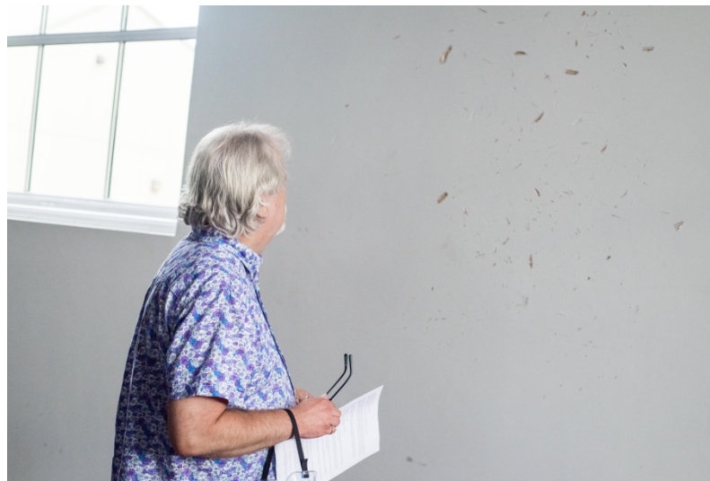
Figure 21: Scratches in wall. August 2019.
