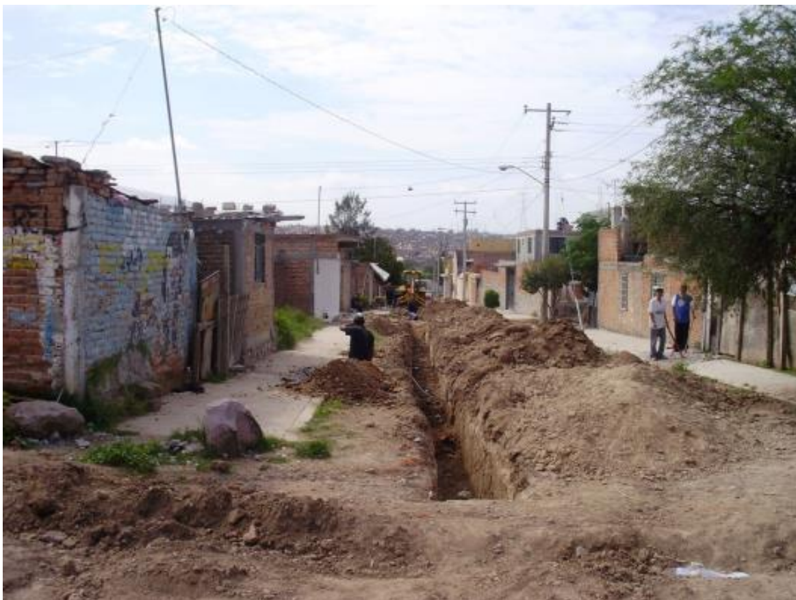
Figure No. 80. Introduction of sewage in El Rocío.
