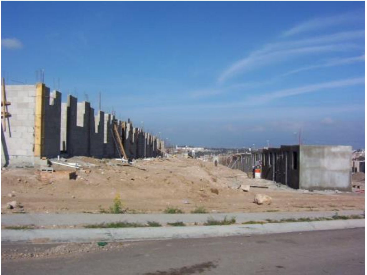
Figure No. 67. Guadalupe Peralta development under construction –note the size of the units and the limited area for expansion.
