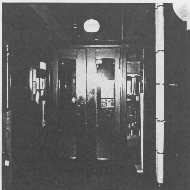
Screen added across ground floor corridor. Note heating pipes to right hand side for radiator system.
