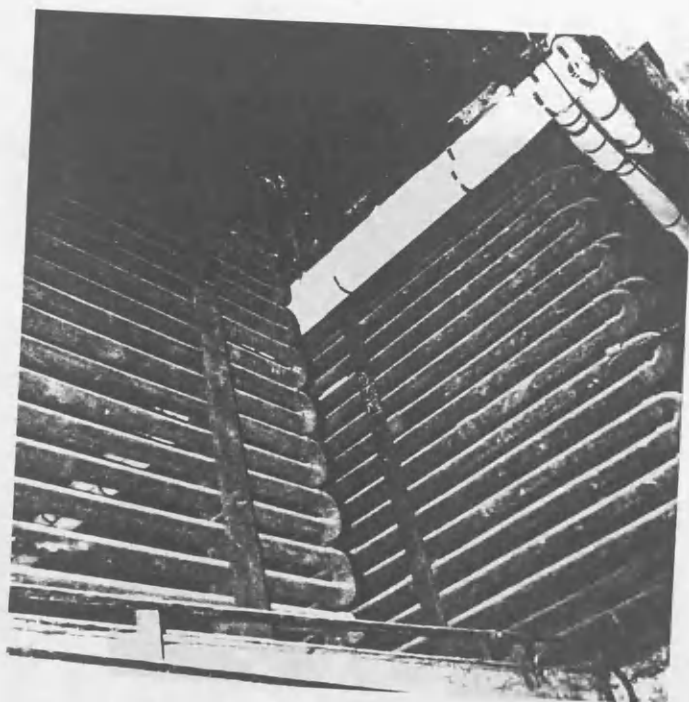
View up into steam coil chamber from fan chamber.
