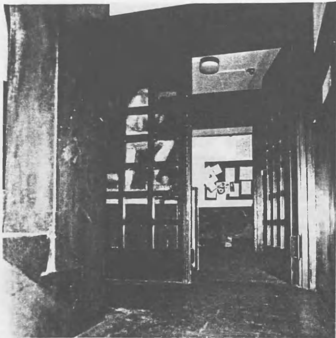
Screen added to West Stair at first floor, separating spaces which originally flowed together. Note replication of original detail, poorly proportioned.
