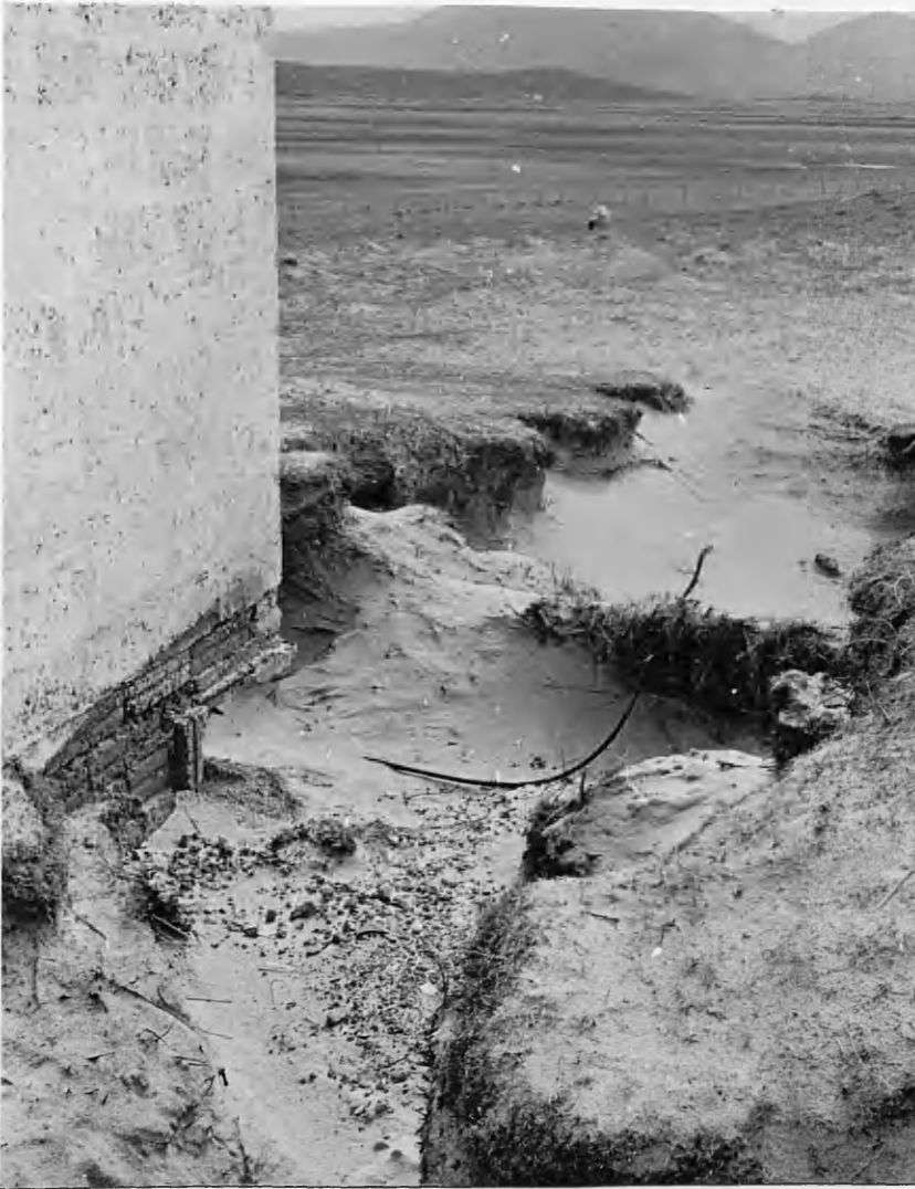
Plate 39. Corridor blow-out running at right angles to the shore through the line of dunes, undercutting a recently built concrete building. Disturbance associated with laying a telephone cable (seen running through the blow-out) may have been the initiating agency. (West Geirinish, South Uist)
