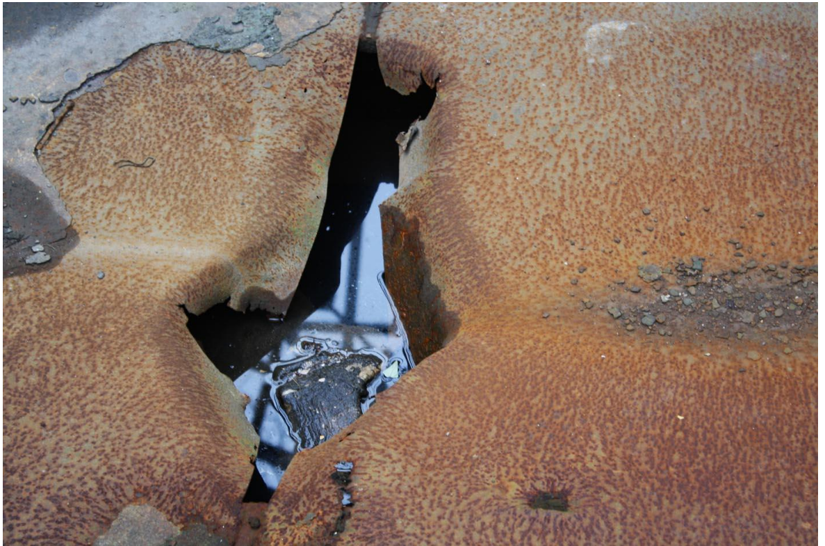
Fig. 02 Surface and Depth: Cracks underfoot in the Graving Docks ruined Pump House (Image: Olden, R.)
