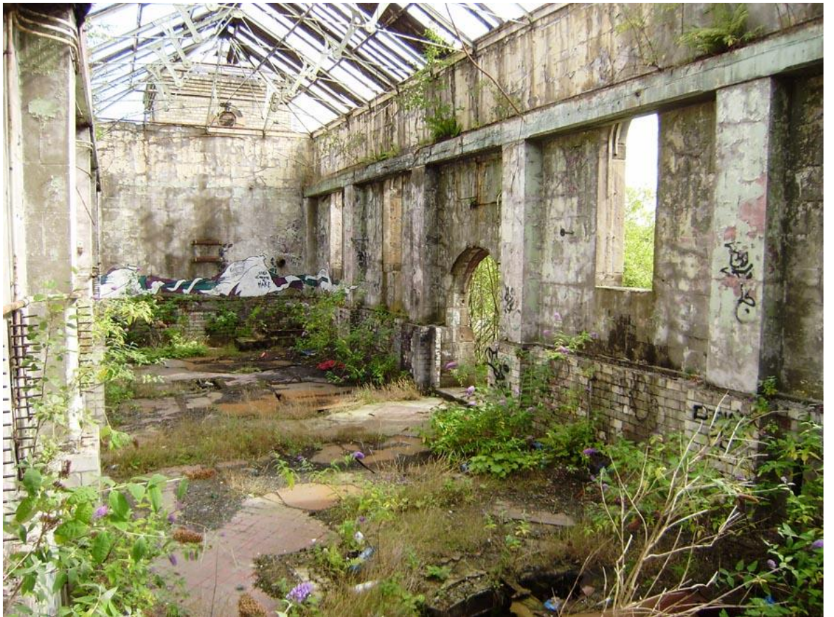
Fig. 03 Dereliction: Shell of the pump house, open to the elements ( Image: Olden, R. )
