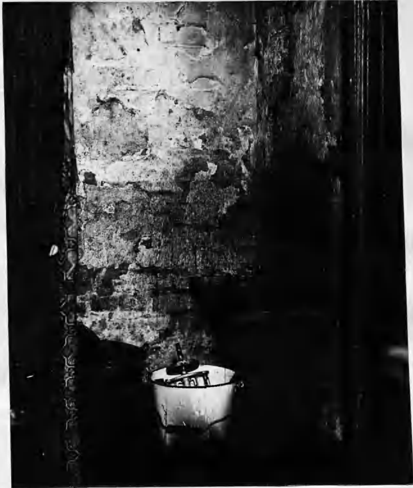
10. A recess in a shop over cellar head where heating of ice-cream mixture is done. (No 22 in Table 2).
