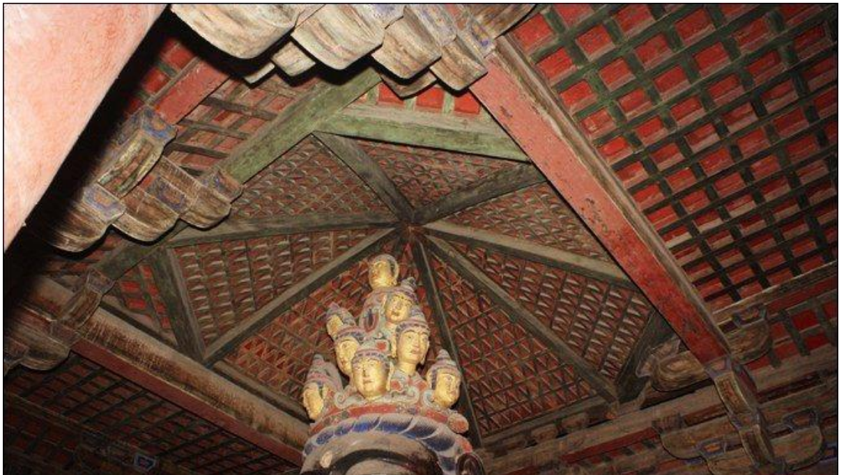
Figure 218 The caisson ceiling, Liao (984) The Guanyin Tower of the Dule Temple, Jixian, Tianjin city
