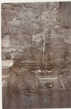
Tap over slop-sink.
