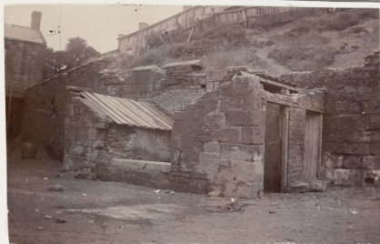
Broken-down Ash-pit. The slops are thrown on the ground, as there are no sinks.
