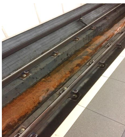
Figure 104 - Photograph of BIOX blooms on the Kelvinhall Subway track.
