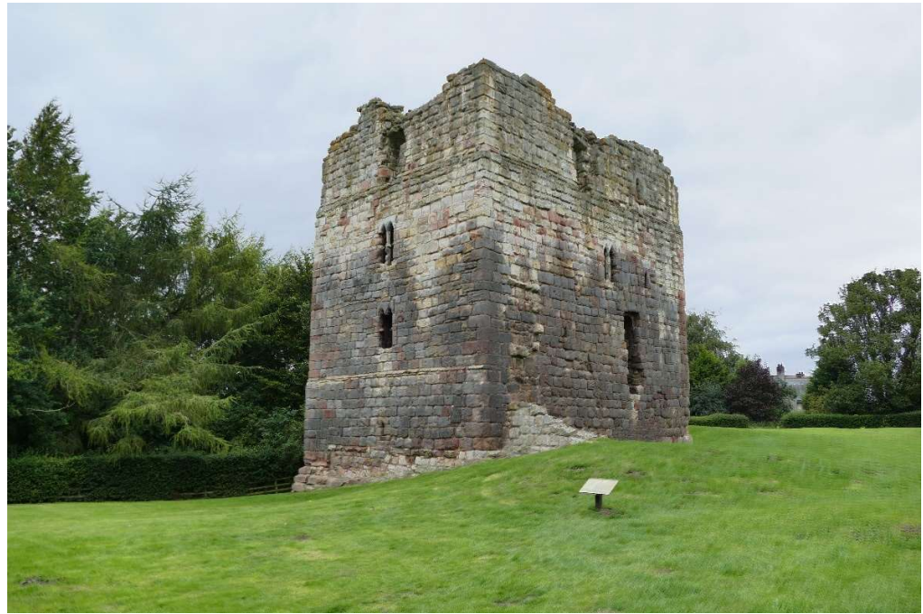
Figure 65 The northwest tower at Etal castle as shown from the south (west and south faces visible). O.B. Goulet-Paterson 2018.
