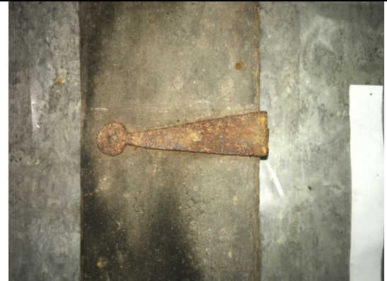
Figure 62. Metal Workers' forged hinges showing active corrosion (red)
