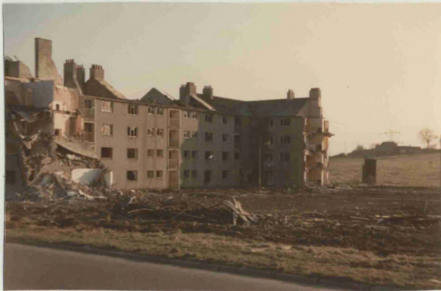
PLATE 9: Demolition in progress at Dunskaith Street, Rogerfield, Easterhouse. These houses had been severely difficult to let. Note that they were four-storey tenements suggesting higher density than normal for the scheme as a whole.
