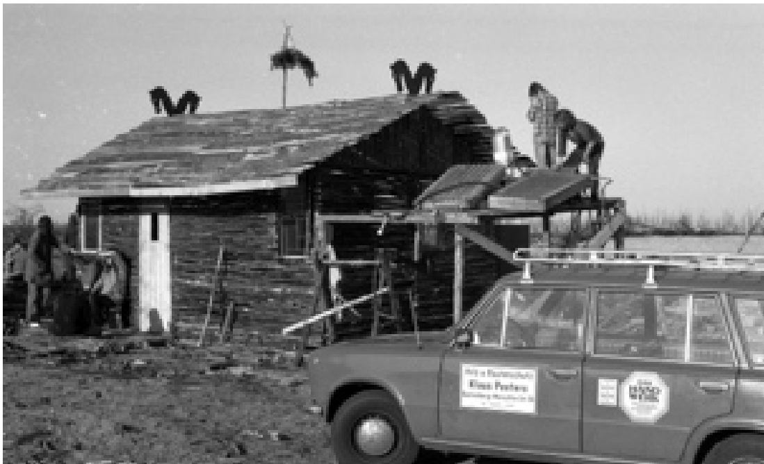
Figure 24 – The installation of solar panels on the roof of one of the buildings on the Free Republic of Wendland (Gorleben Archiv, 1980p)
