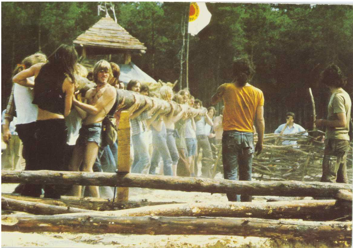
Figure 19 – Activists in the FRW carrying a large tree trunk together for the construction of village structures (Gorleben Archiv, 1980a)
