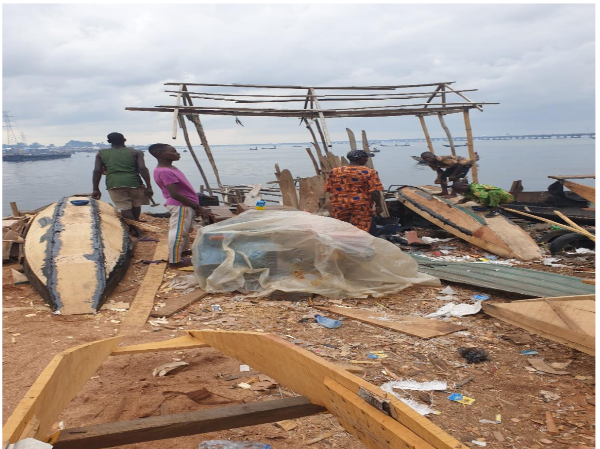
Figure 9: Building a workshop in the middle of the water (Source: Author's file)
