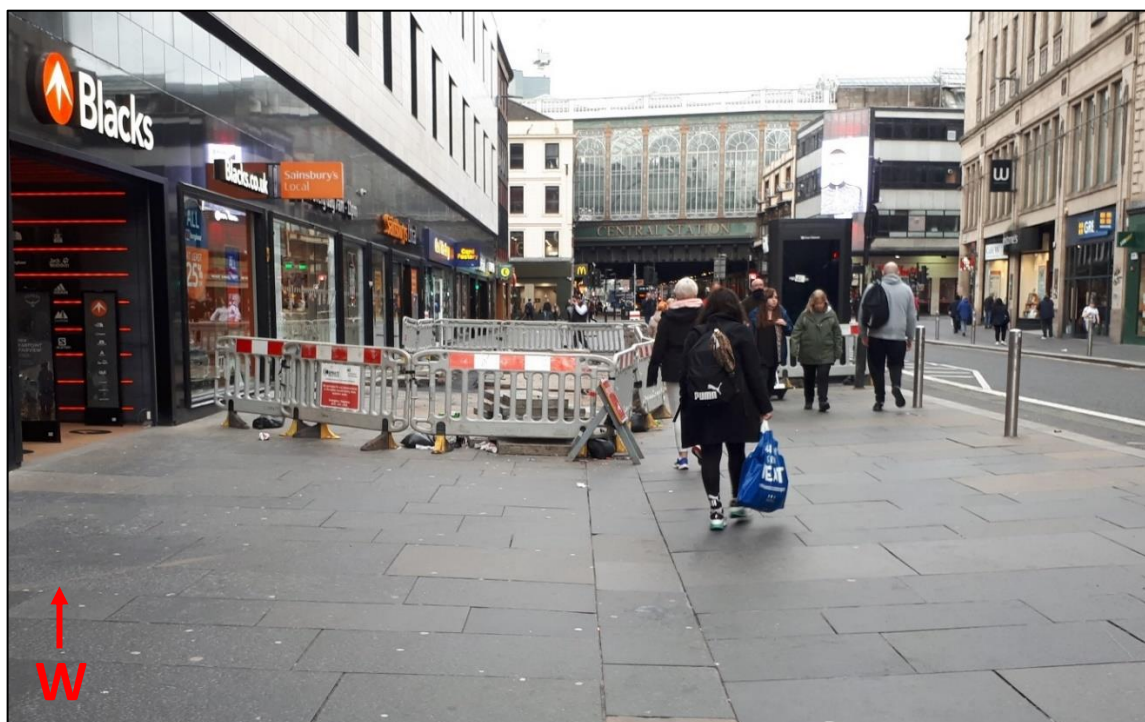
Figure 80: Pinch point control site 2 on Argyle Street where construction works forced people to walk either through a small gap between the barriers and advertising screen, or into the carriageway. Image © author.
