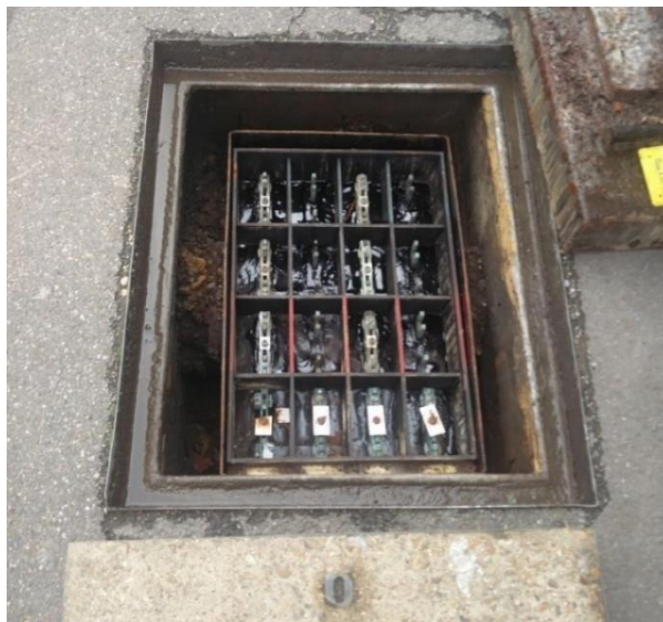
Figure 1.5.7: Four-way LV linkbox showing two solid ways and two open ways in Hounslow, London.
