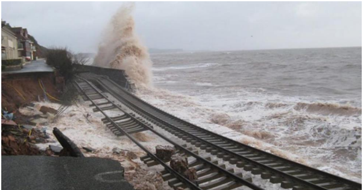
Figure 3-2 Collapse of Dawlish sea wall in February 2014
